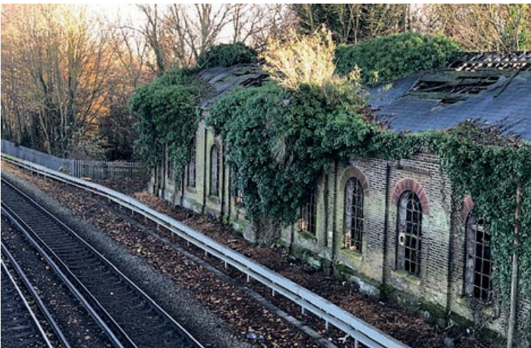
The engine shed at Faversham (a grade II heritage at risk listed building)
