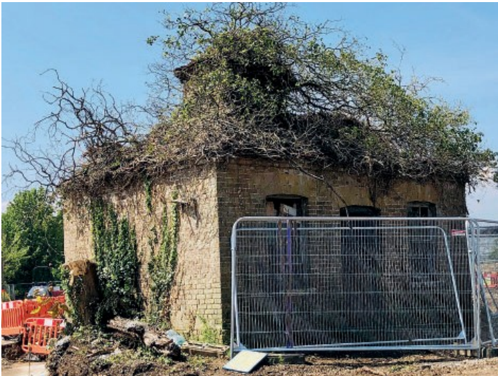
The Proof House at Marsh Gunpowder Works awaiting repairs and restoration summer 2019 ( a grade II listed building).
