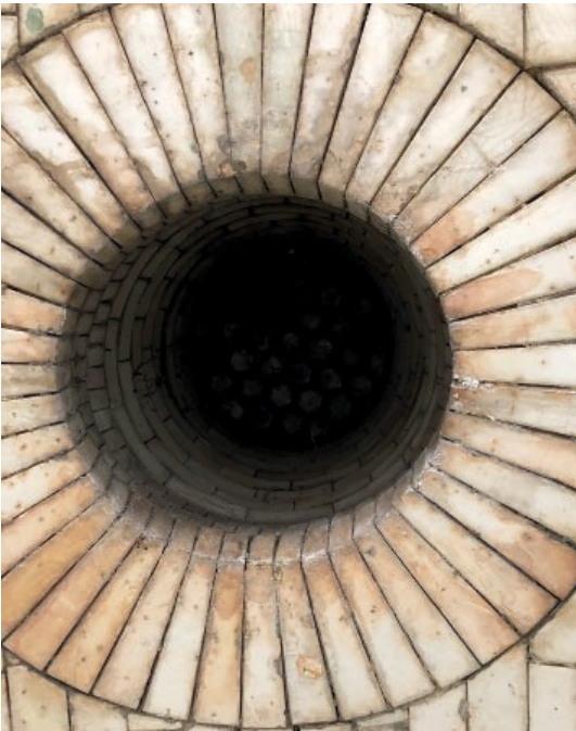
Tiled underpass feature at Faversham Station (a grade II heritage at risk listed building).
